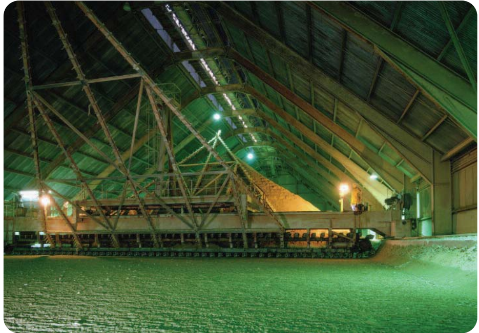
Clay/Limestone Store showing stacker and reclaiming. Max. capacity 43000 tonnes, rail dia. 88m.
